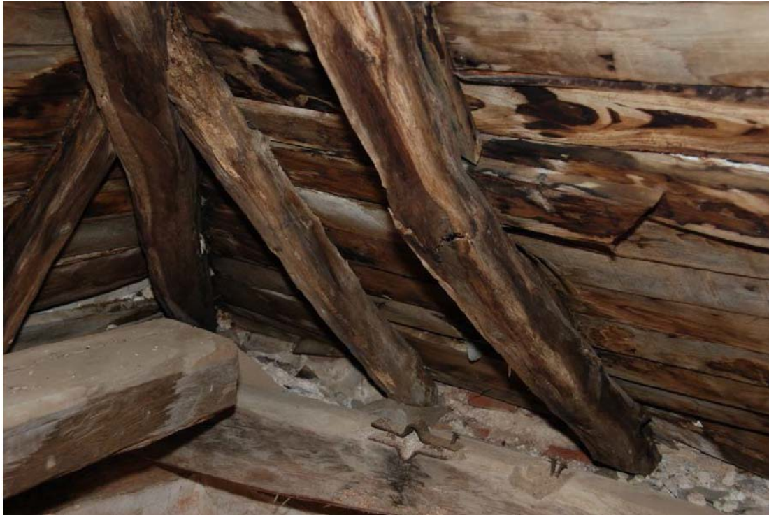
PICTURE 4 – DAMAGE TO THE WOODEN STRUCTURE – STRUT AFFECTED BY DAMP
